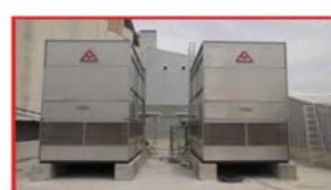
ENCLOSED TYPE / EVAP.CONDENSER
